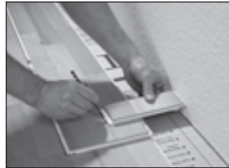
Use a remnant to transfer the wall outline to the last row of planks.
